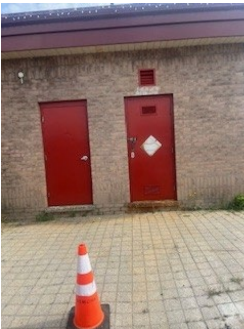
Figure 3 – Summer students completed various painting projects around the City including these doors at the PFC.
