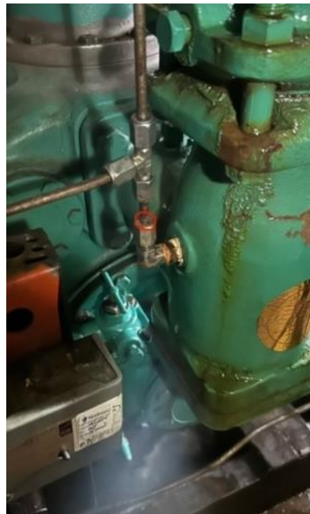
Figure 4 – An Ammonia leak on the head cooling line of one compressor necessitated an emergency repair the weekend prior to opening at the SHSMA. Leak circled in red.
