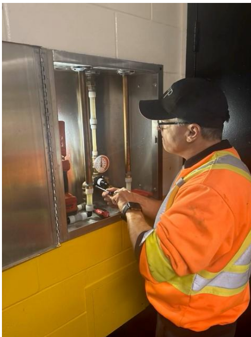
Figure 3 - Robin Imbeau adjusts a mixing valve at the SHSMA.
