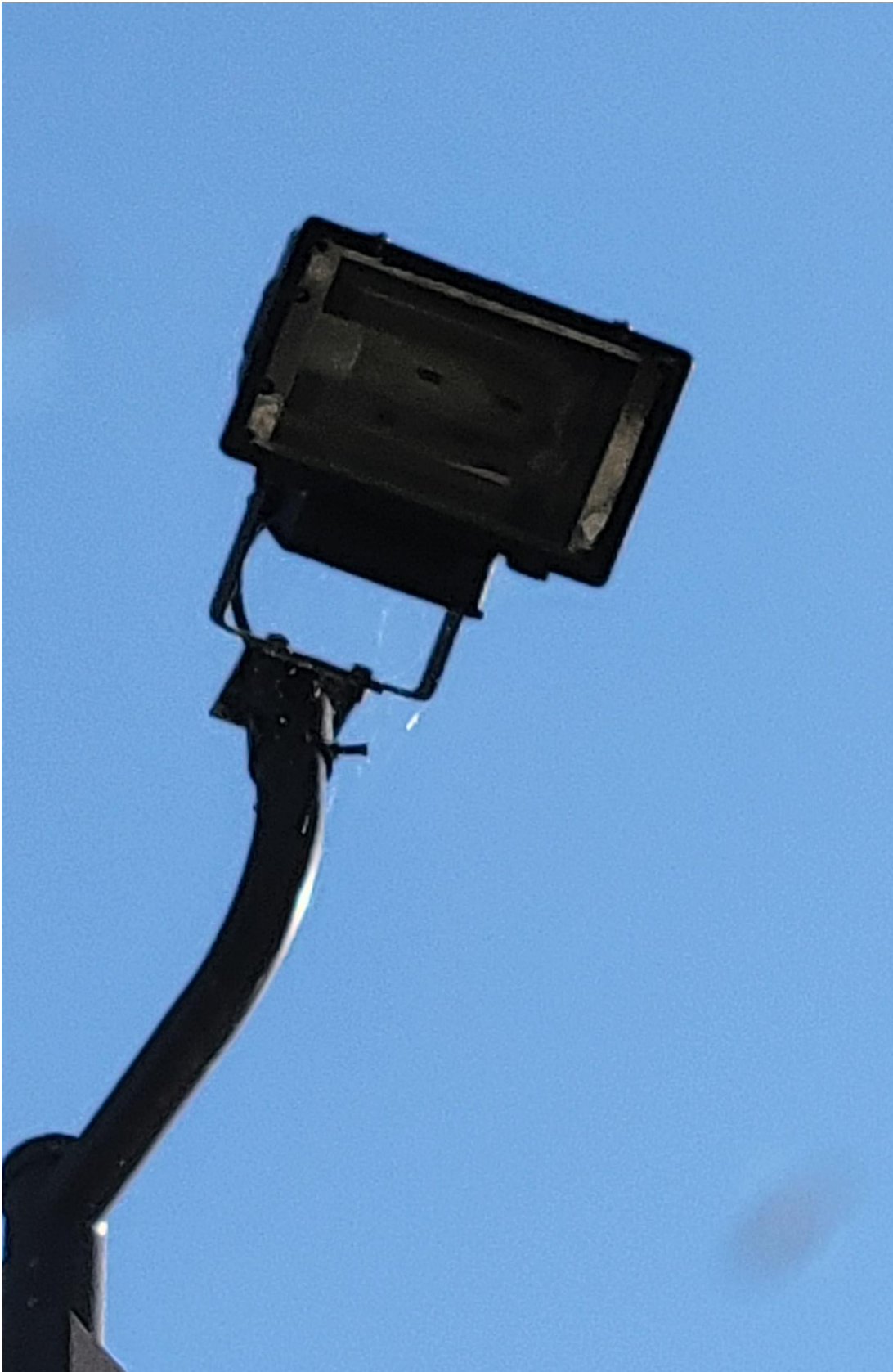
Figure 3 - Close up of existing fixture
