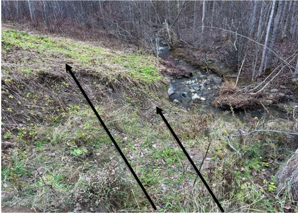
Photo #7 - The slope soil strata: The grass and the eroded silty clay underlay.
