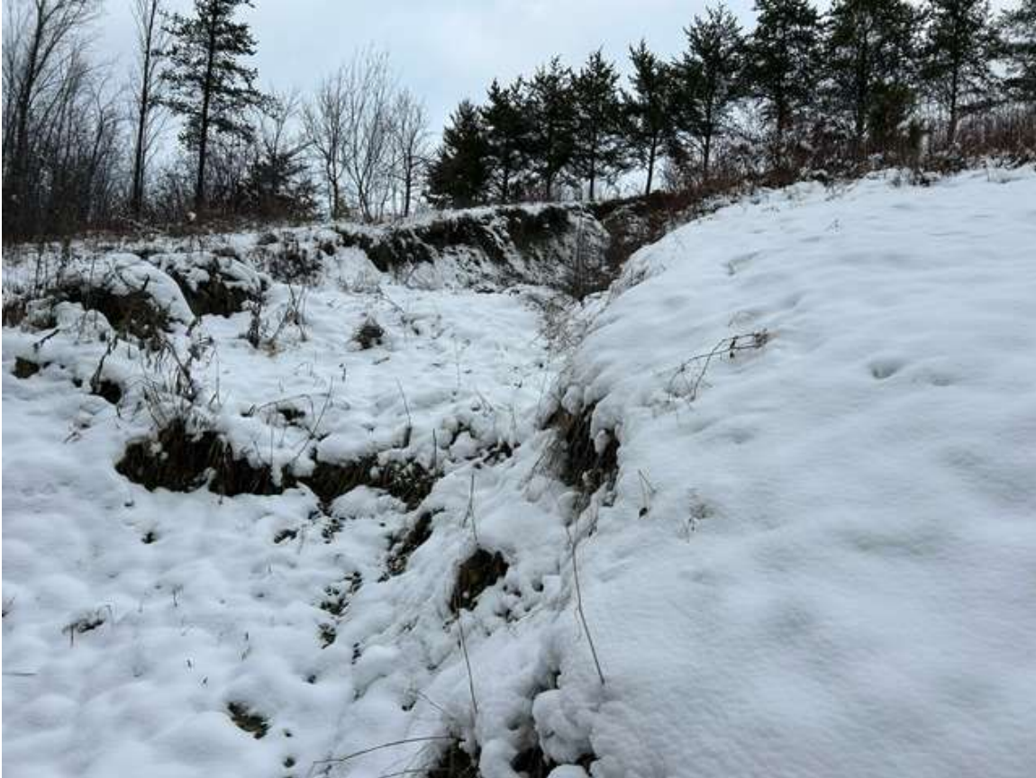
Photo #5- Current Condition of the eroded surface -November 2024.
