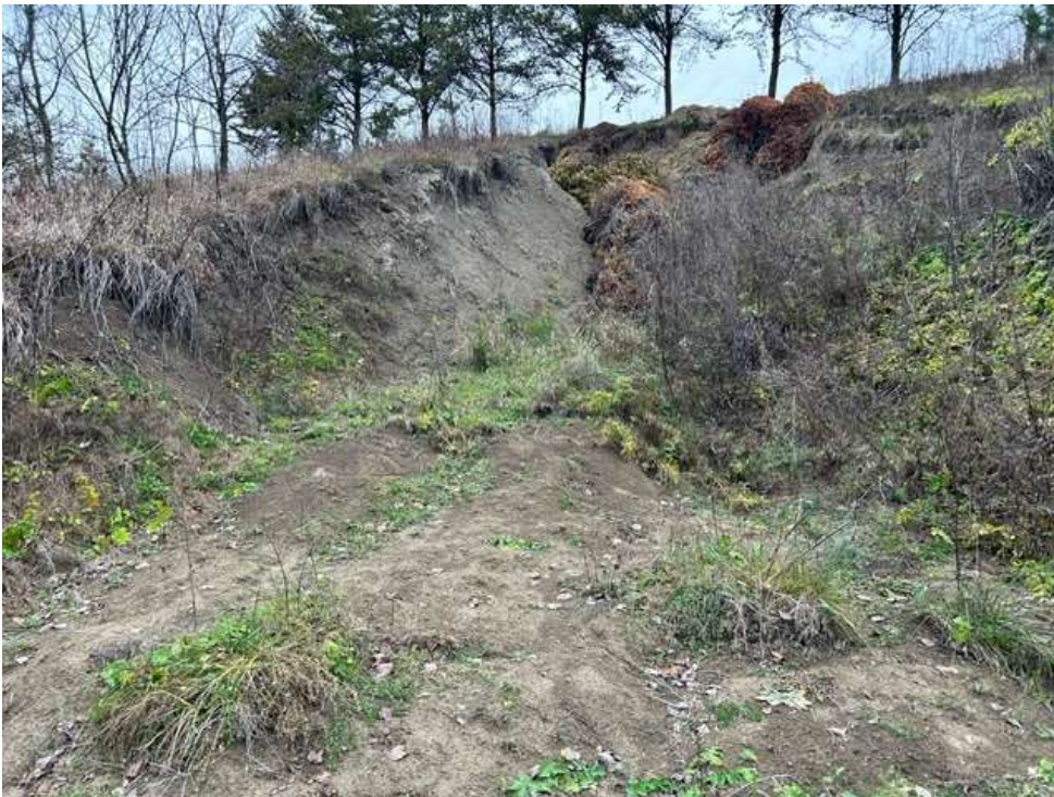
Photo #1-Looking north- The top of the slope with tree line and the wash out.
