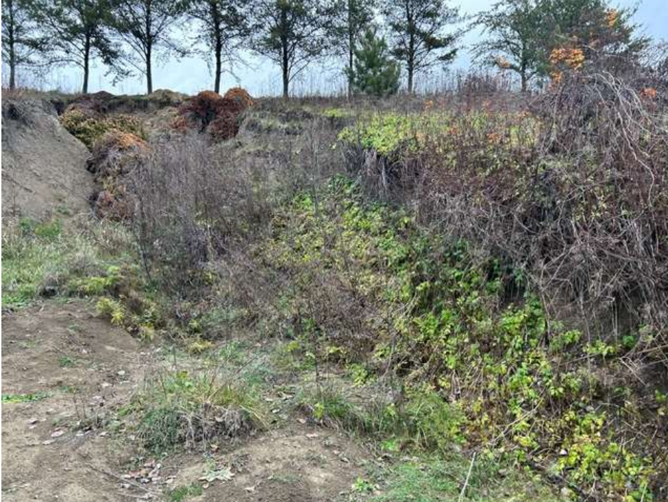
Photo #2 - The silty clay wash out and a gully- August 2024.
