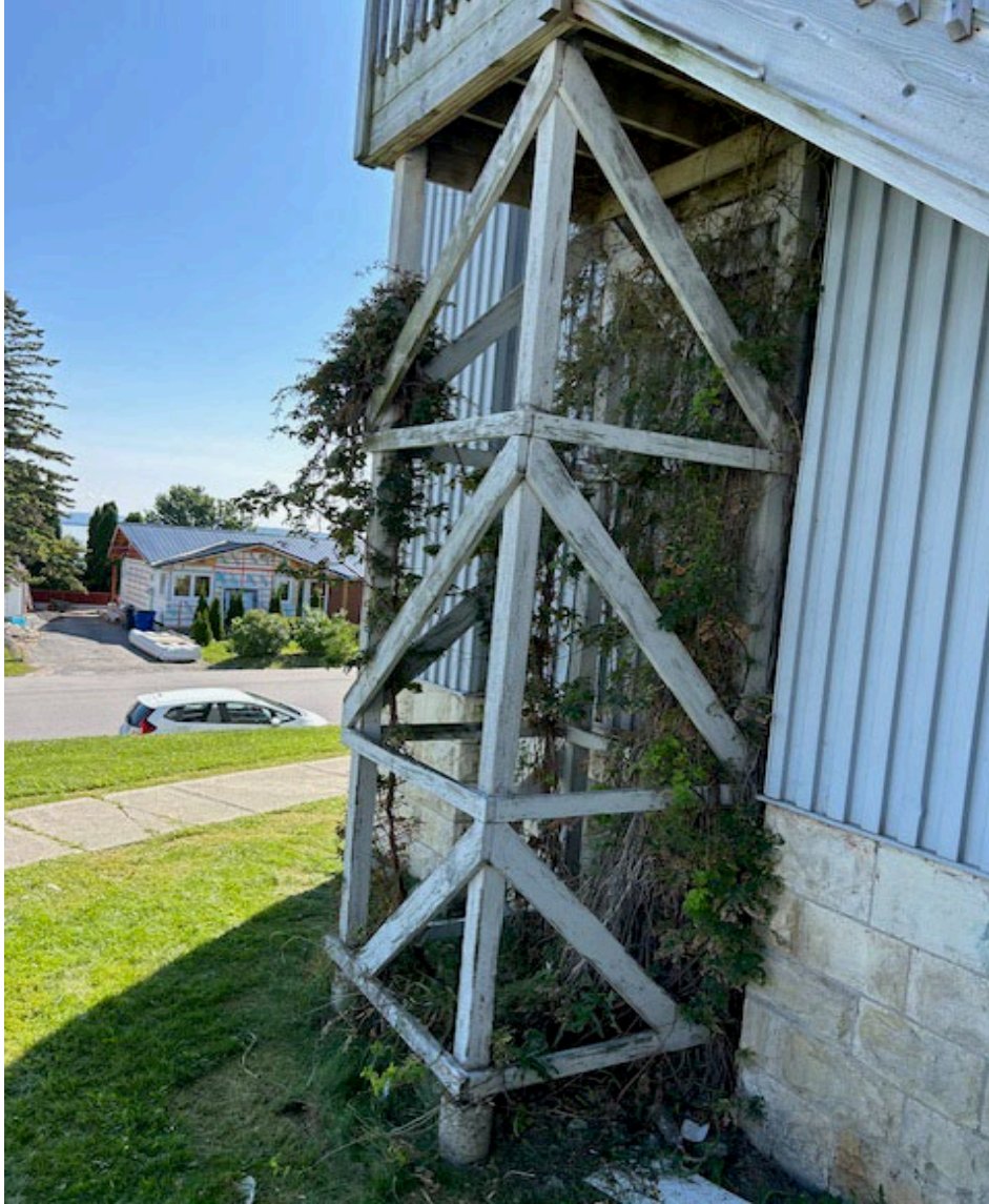
Pier supports – they are lifting
