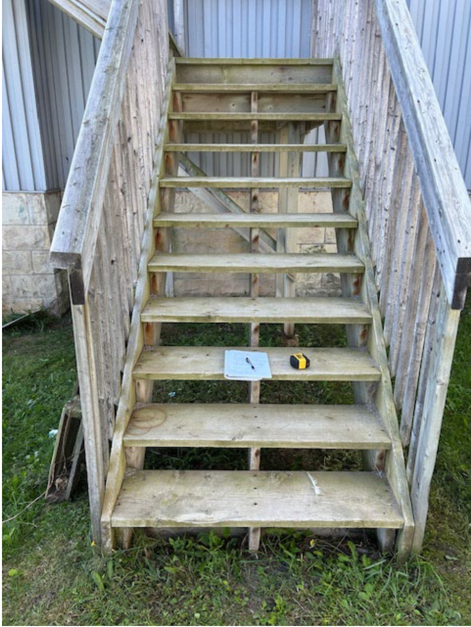
The railings are wobbling
