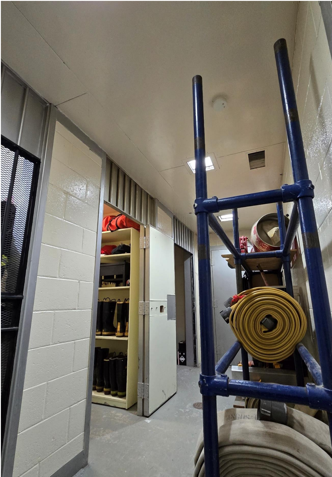
Figure 2 - Photo of hallway outside three jail cells. Ceiling panel material is present in this area and all three jail cells.
